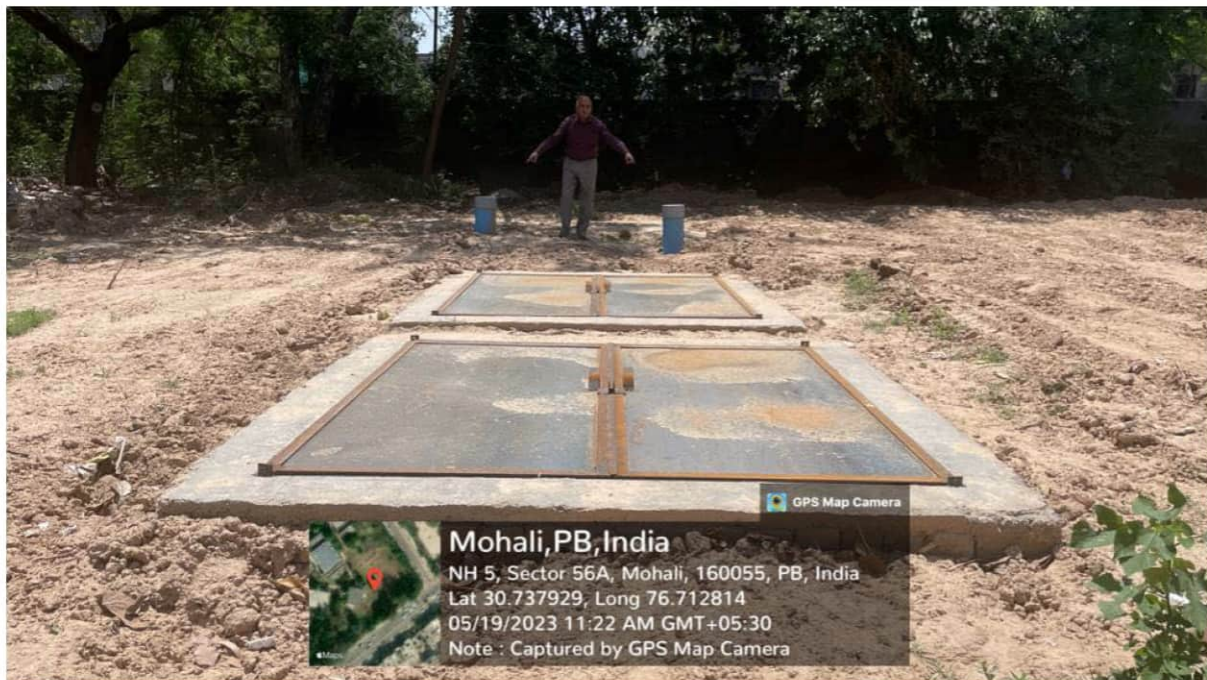
(Fully Functional Rainwater Harvesting System)
